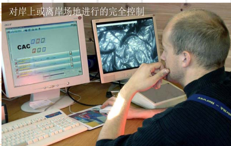
On-line monitoring & operating system
