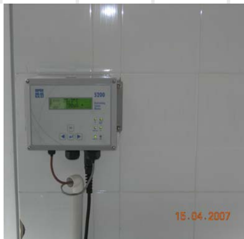
DO, pH, Eh monitoring meter
