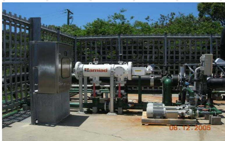
Water treatment equipment in Spain
