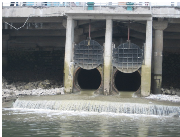
Fig. 8. One of 14 direct discharge outlets along the Yalu River.
